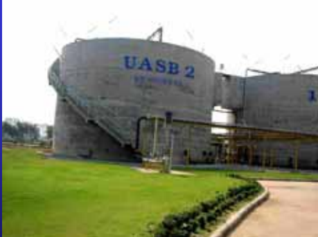
Waste water from the cassava starch factory is converted into biogas to be used for drying the starch
